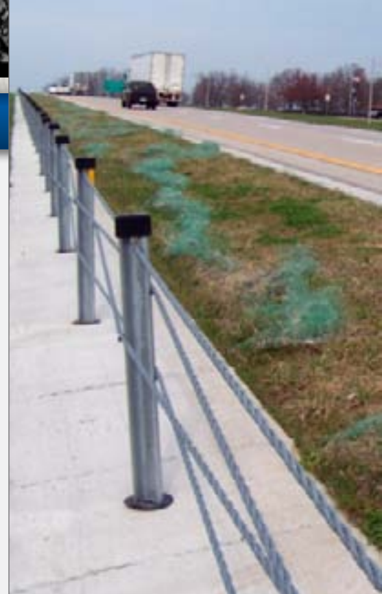
Cable Barrier Project with ECB Issues
